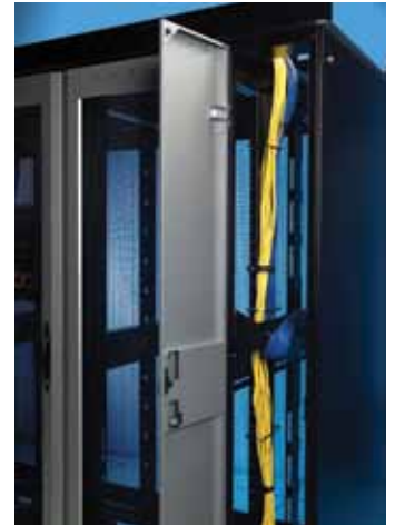
Side cable management channel.
